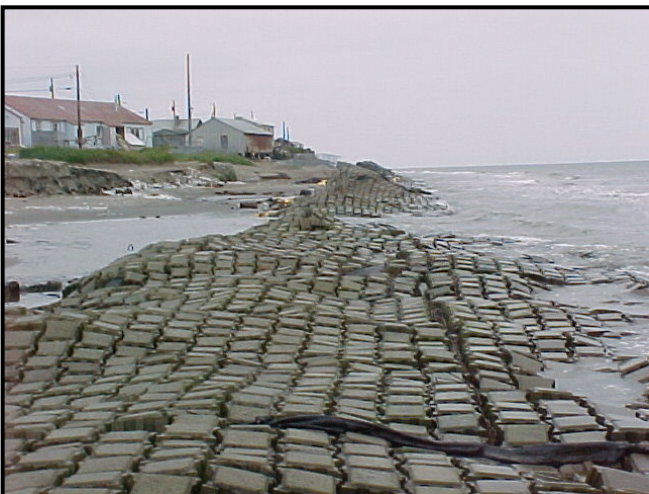
Photo 10: Failed sea wall. (Credit: Brice Eningowuk)
