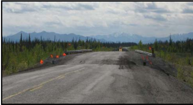
Left: Impacts from thawing permafrost on Alaska Highway north of Beaver Creek (Source: Prof. Billy Connor, University of Alaska Fairbanks 2009, Permafrost and the Alaska Highway) Below: Storm surge undercutting western Alaskan coast (Source: IAWG Final Report)
